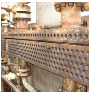
FinFan cooler before a maintenance
